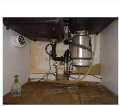
Disposal not operational
